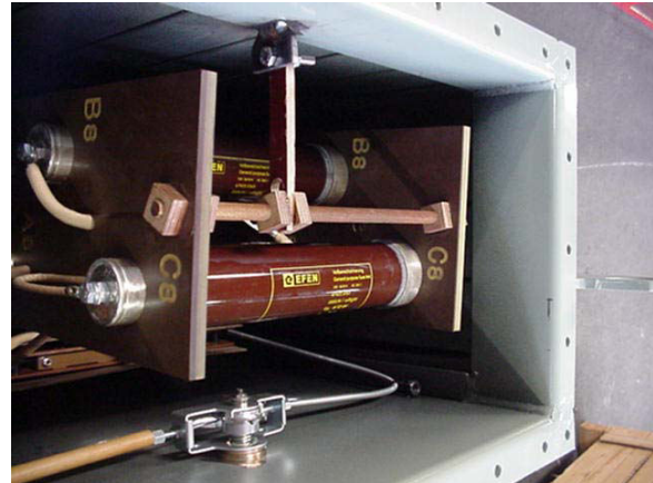
Fig. 4: Under-oil m.v. back-up fuses in a transformer tank
