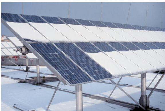
Fig. 3.2: Solar generator partially covered by snow
