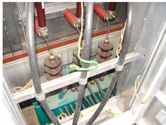
Figure 13: Example of not insulated places in a transformer substation
