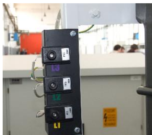
Figure 2: Voltage indication on VOH 01 carried out with IN5
