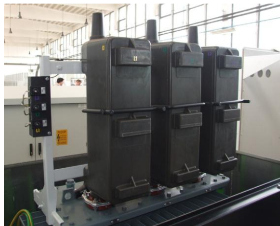
Figure 1: Insulated HV fuse holder VOH 01 (design by TSN) mounted on a transformer's cover (50 kVA).
