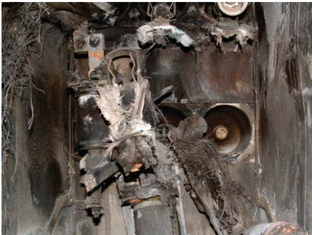
Fig. 1: destroyed medium voltage switchgear as a result of a blown-up HH-fuse
